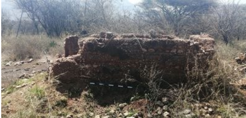
Figure 65 – Intact walling of the poorly preserved historic homestead (this one is the best preserved of the locality).
