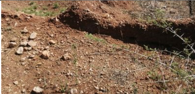
Figure 49 – Walling next to the weathered rubble of washed away walling, bits of concrete are visible.
