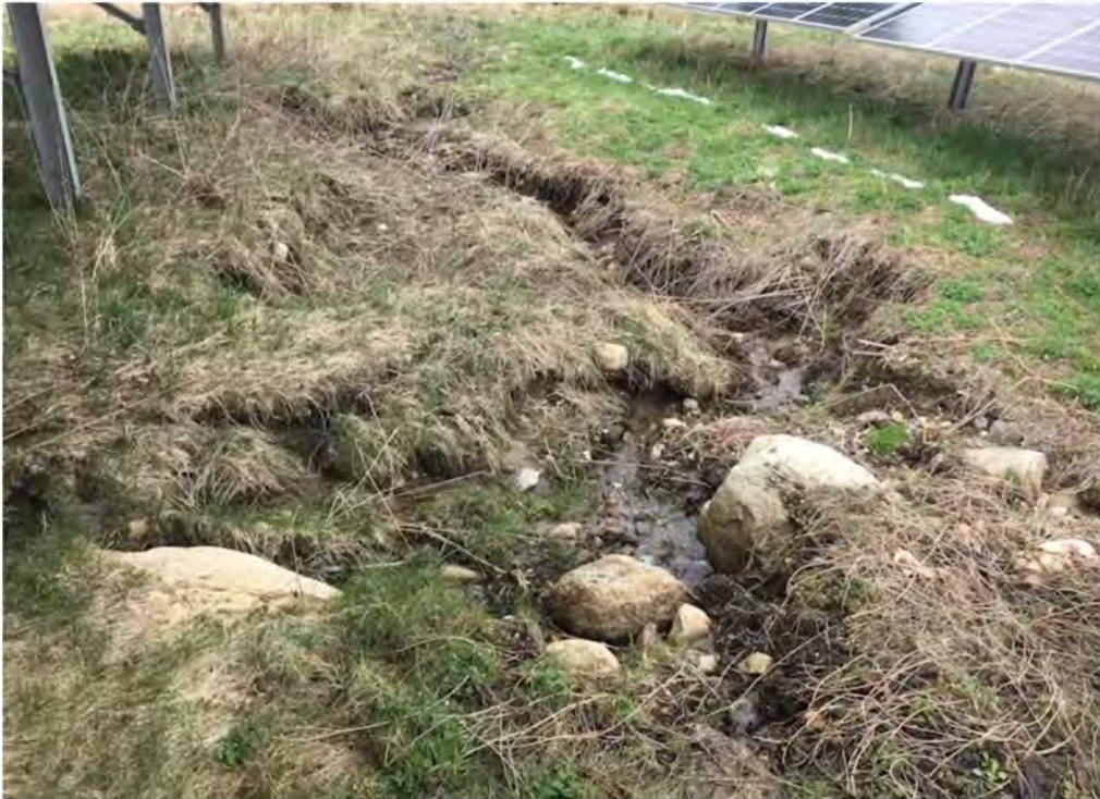
Figure 6-5: Eroded channel caused by concentrated stormwater flow (DaPonte, et al., 2020)
