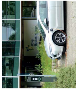
Electric company car charging at Amersfoort office
